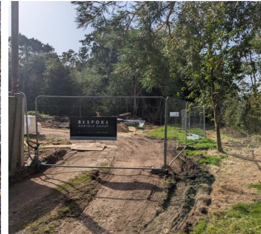
Fence over public land for approx. 4 months
